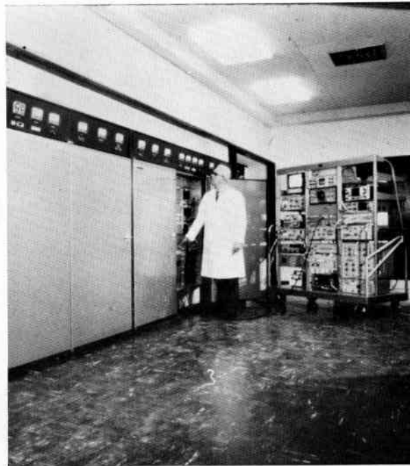
Crystal Palace transmitter hall showing a UHF test trolley in use. Normally the station is unmanned
